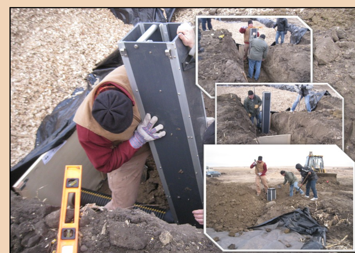
5. Installing the drainage control structure used to divert water through the trench.
