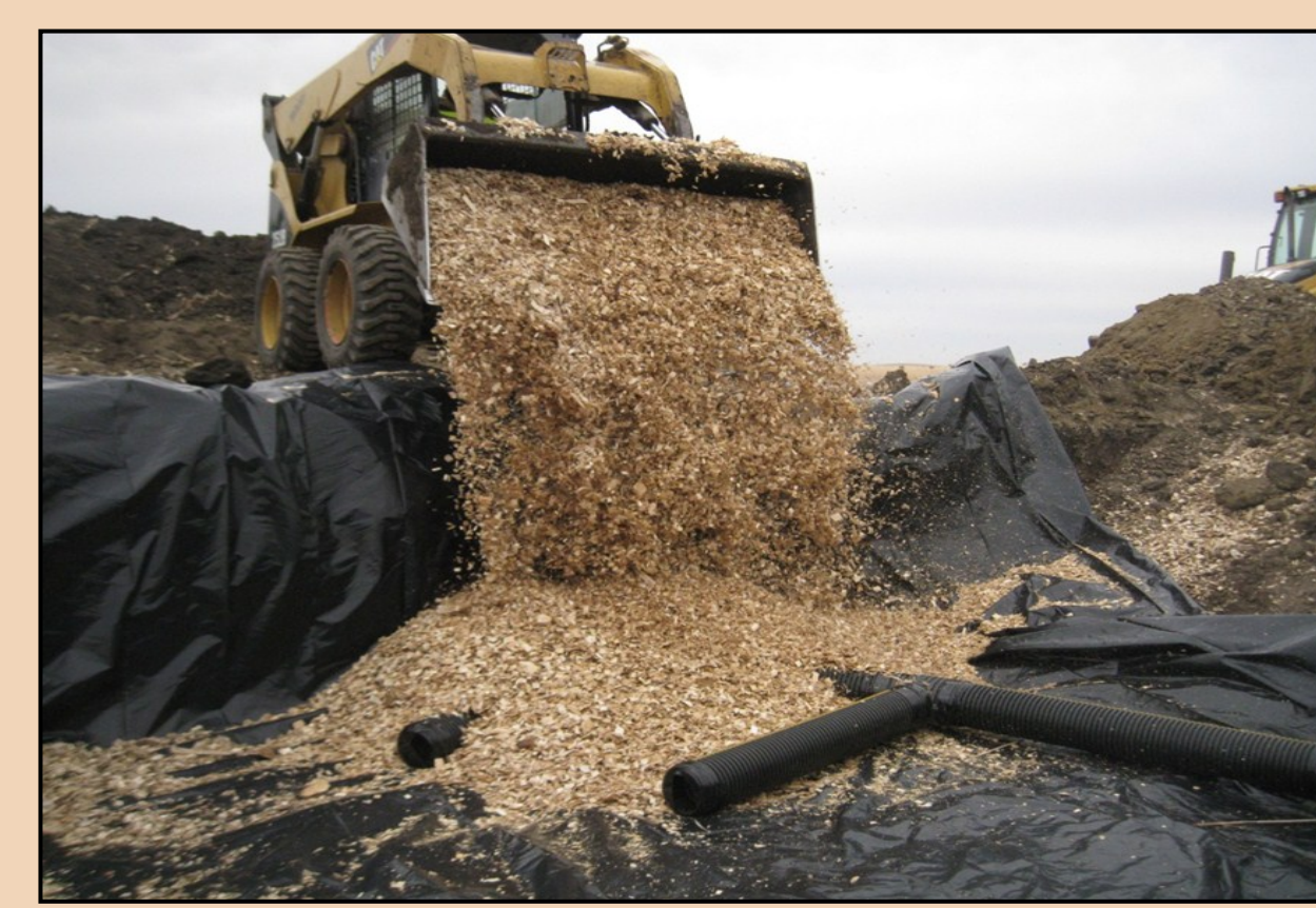
3. Filling the lined trench with woodchips. Perforated PVC distribution/collector manifolds were placed at both ends.
