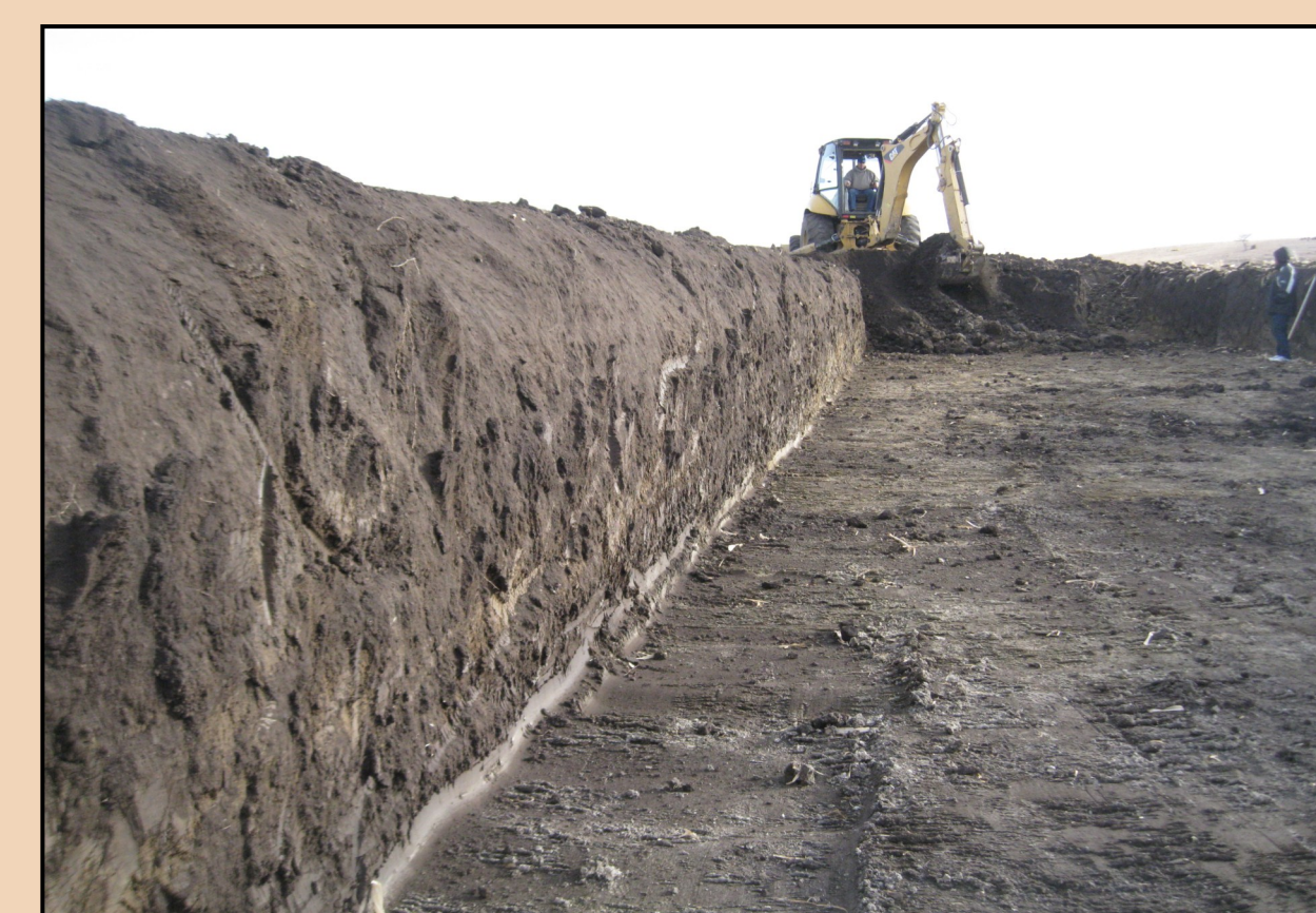
1. Excavating the trench about 21 ft. wide, 130 ft. long and 5 ft. deep for the bioreactor.
