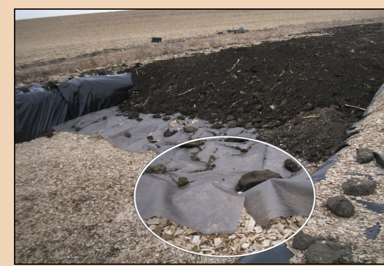
4. Covering the woodchips with a geo-textile fabric to prevent the woodchips from being contaminated by the soil.
