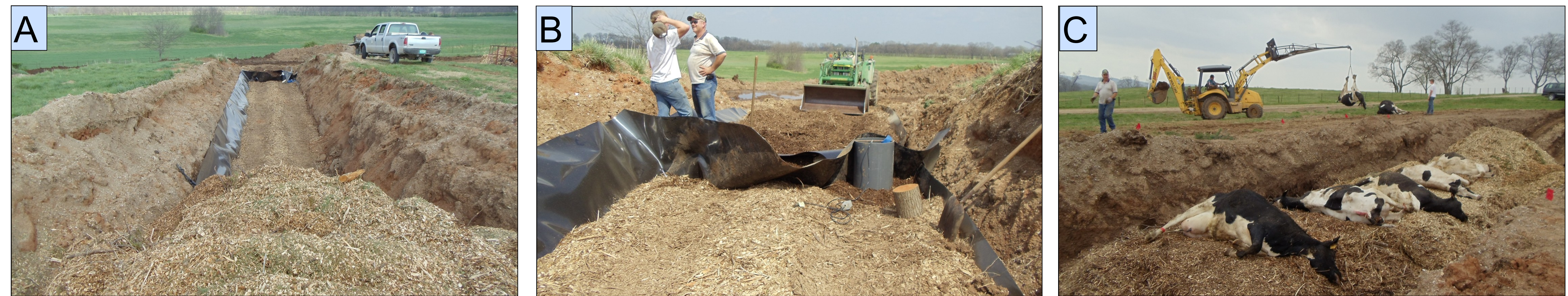
Figure 1. A. Finished burial trench. B. Close-up of leachate collection sump. C. Placing the carcasses in the trench (April 11, 2011).
